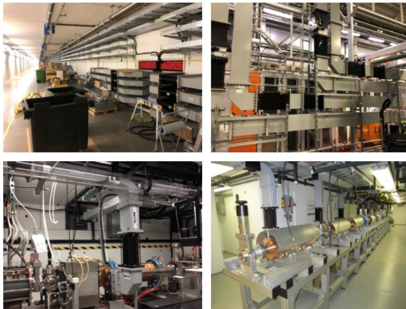
Waveguide “runs” of flexible and rigid sections in high-energy physics laboratories
